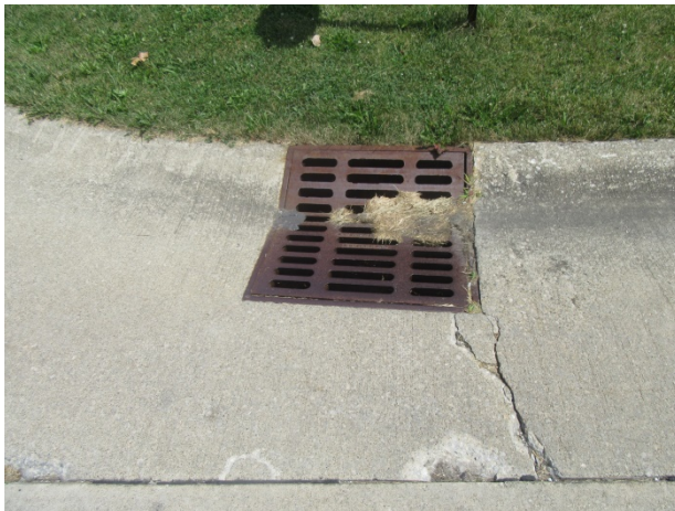
Catch basin collar crack at Horseshoe Drive
