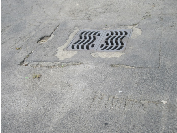
Catch basin deterioration at Morgan Court
