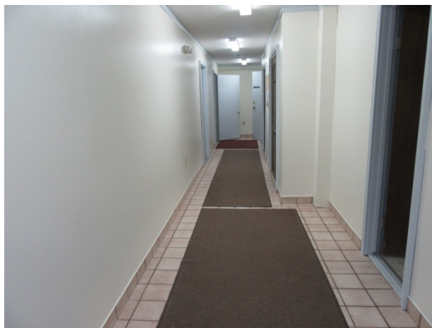
Ceramic tile at the office building hallway; we note isolated deterioration
