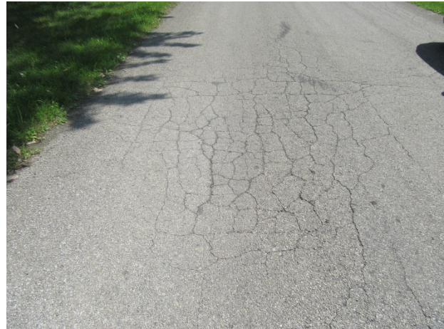
Phase 1 pavement, cracks at Sunset Drive
