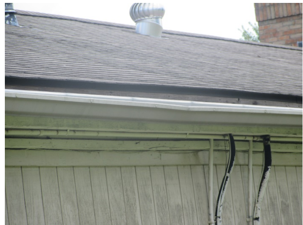
Minor gutter deterioration at the office building
