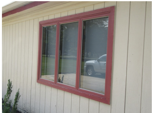
Window; we note finish deterioration
