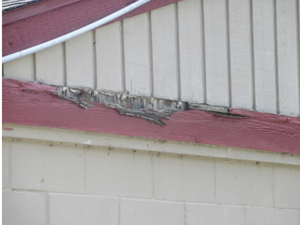
Trim deterioration at the office building
