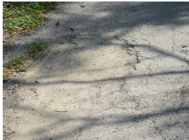
Phase 2 pavement, deterioration at Bass Court
