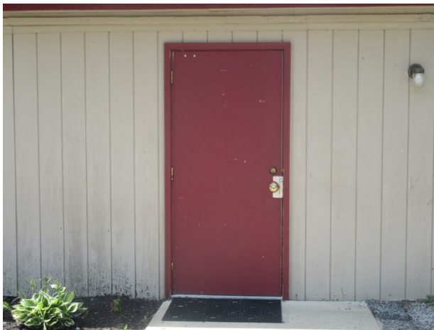
Door; we note finish deterioration
