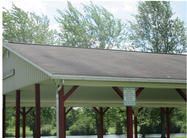
Pavilion roof; we note shingle lift
