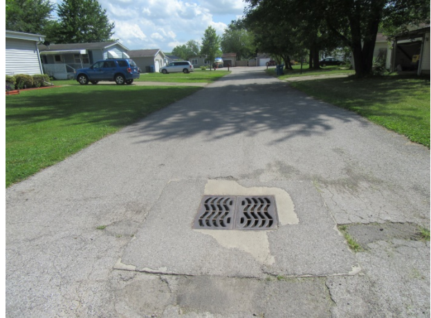
Catch basin exposed collar at Pike Court
