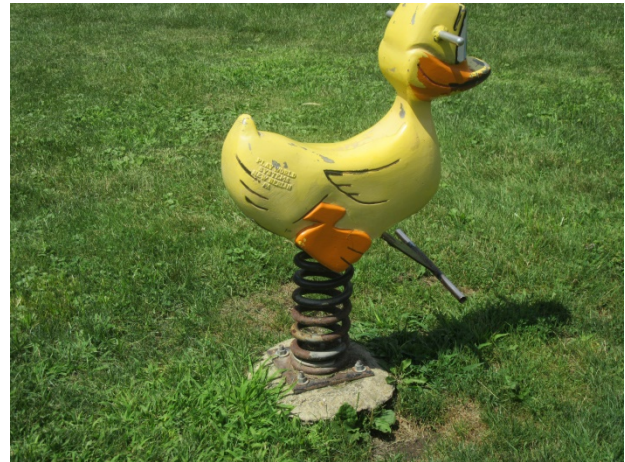
Spring rider rust and finish deterioration
