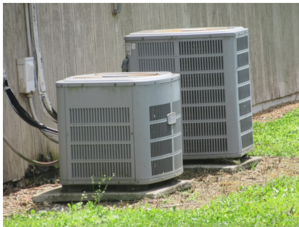
Office building condensing units
