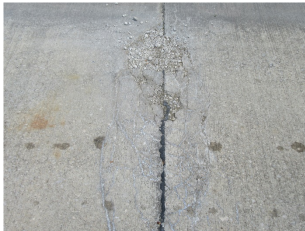
Concrete street deterioration at Horseshoe Drive
