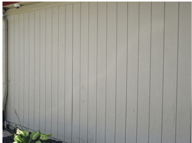
Plywood siding paint finish deterioration at the office building
