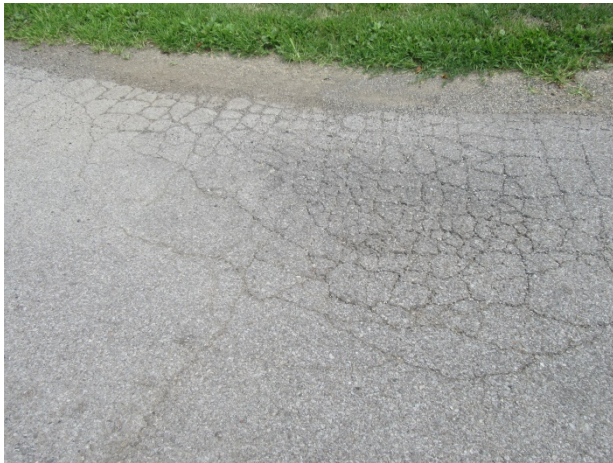
Phase 3 pavement, cracks at Hickory Run
