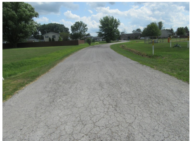
Phase 5 pavement, cracks and deterioration at Ringneck Court
