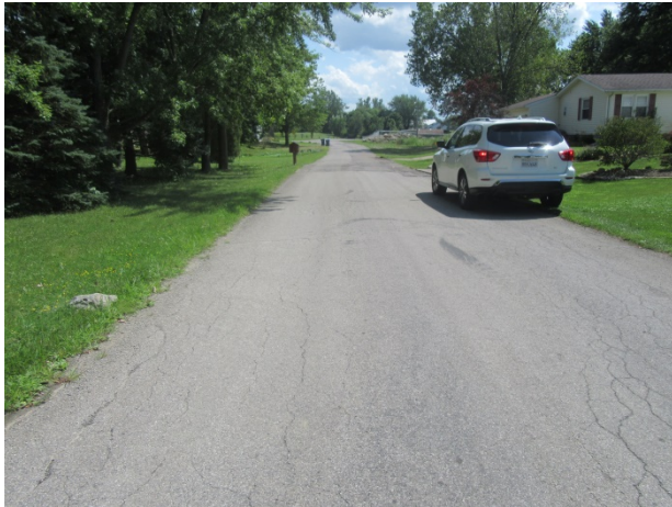
Phase 1 pavement, Sunset Drive; we note cracks
