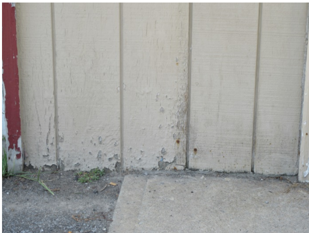
Trim and plywood siding finishes deterioration at the office building
