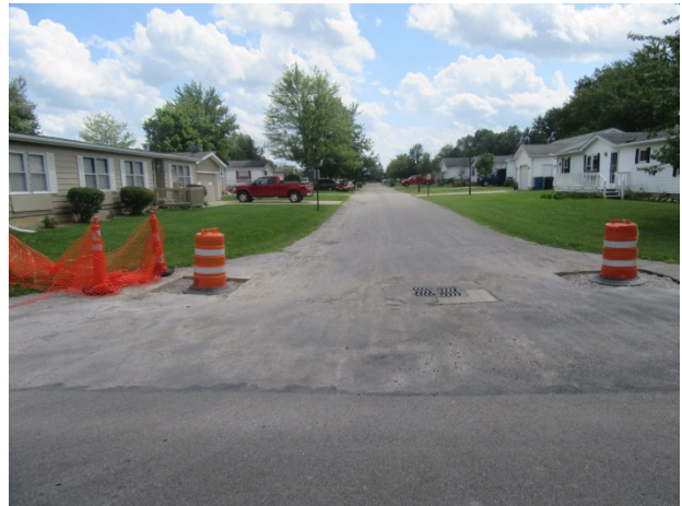
Phase 4 pavement, ongoing repairs at Stallion Court
