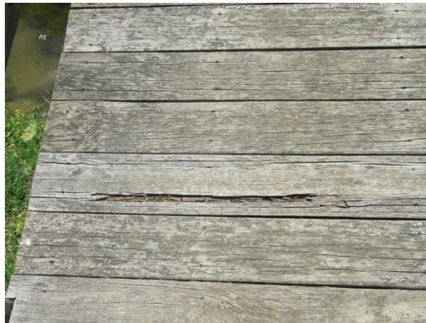
Wood bridge deck board deterioration
