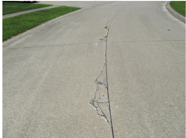
Concrete street deterioration at East Lake Court
