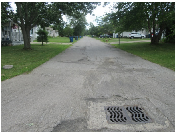
Phase 5 pavement, Palomino Court; we note cracks and deterioration
