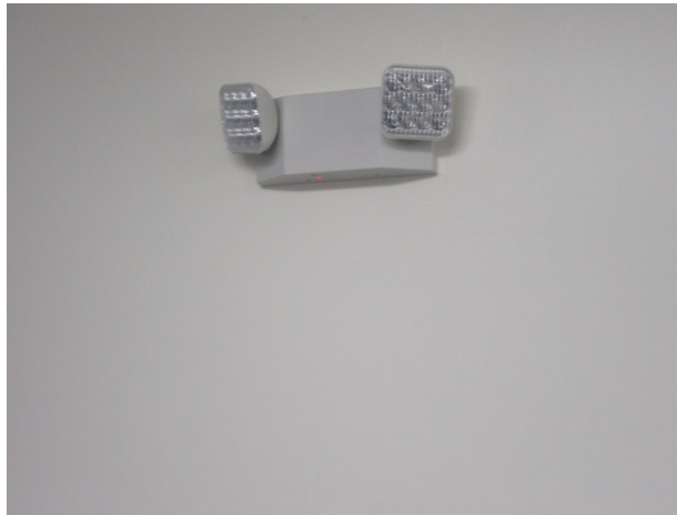
Emergency light fixture
