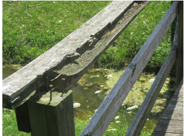
Wood bridge railing deterioration and loose fasteners
