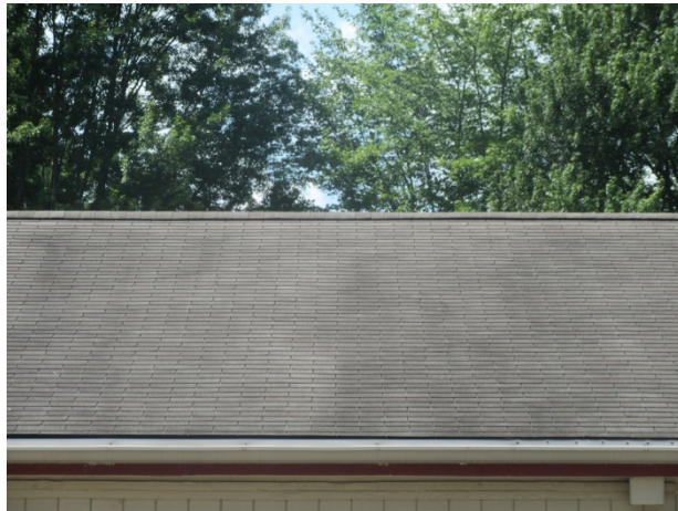
Maintenance building roof; we note shingle discoloration
